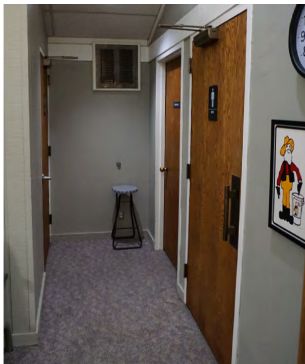
Public restroom access via blind corridor
