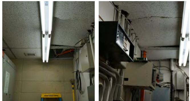
Damaged ceiling tiles with exposed wiring
